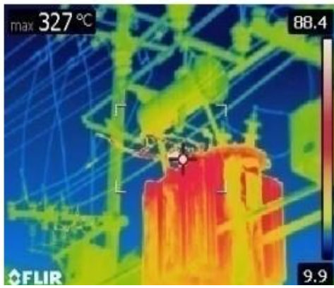
Figure.3. Hot spot on line joint and transformer [17].
